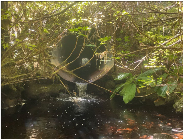
Figure 2.—Perched culvert at waypoint 1000.
