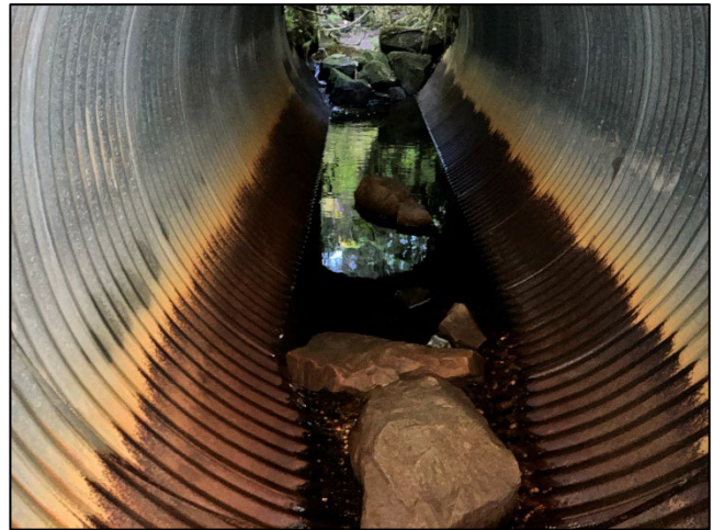
Figure 3.—Inlet of culvert with fallen rip rap blocking the channel and fish passage at waypoint 1000.
